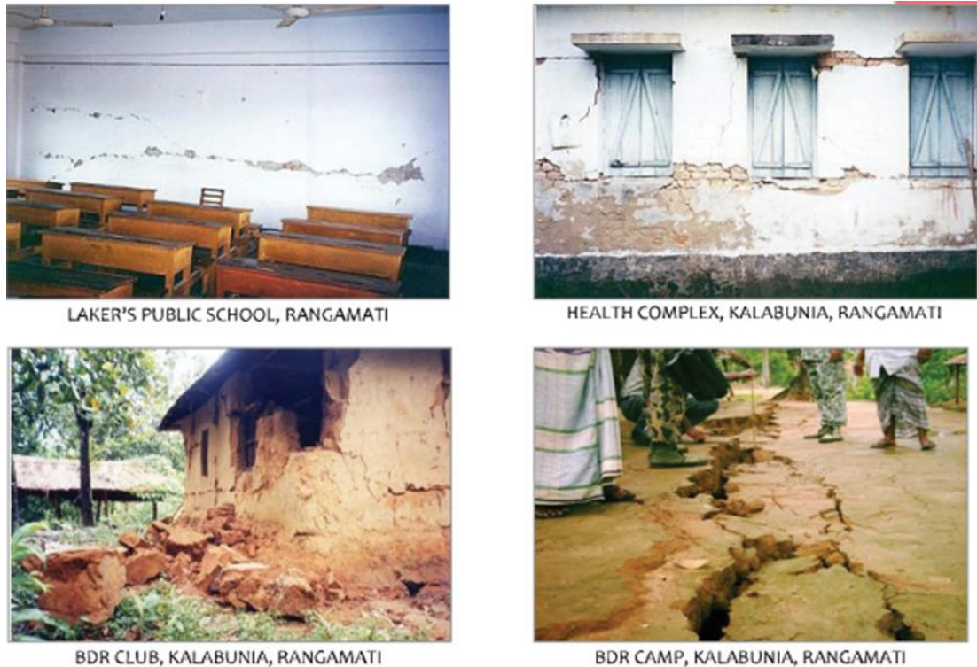
Figure 1.4: Damage of earthquake in Kolbunai, Rangamati after 2003 earthquake
